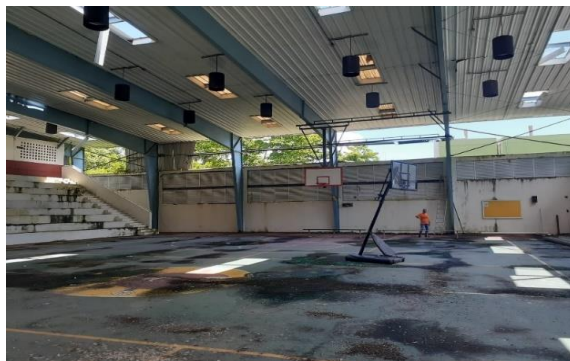
Figure 2. Photograph of Physical Education Facility at Escuela Superior Doña Fela in Yabucoa taken after Hurricane María struck the island. Taken in 2018 by Edwin Ortíz and Gabriel Fontanez
