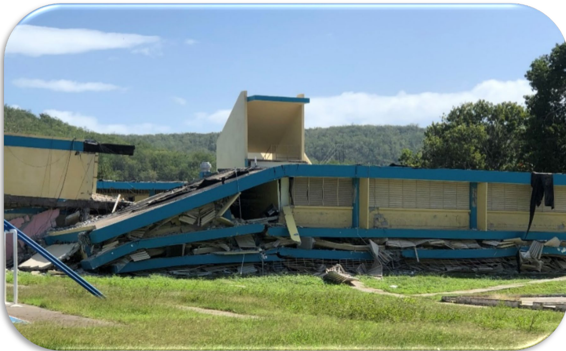
Figure 4 : Collapse of Agripina Seda School in Guánica due to January 7, 2020 Earthquake (Pacheco-Crosetti, 2020).
