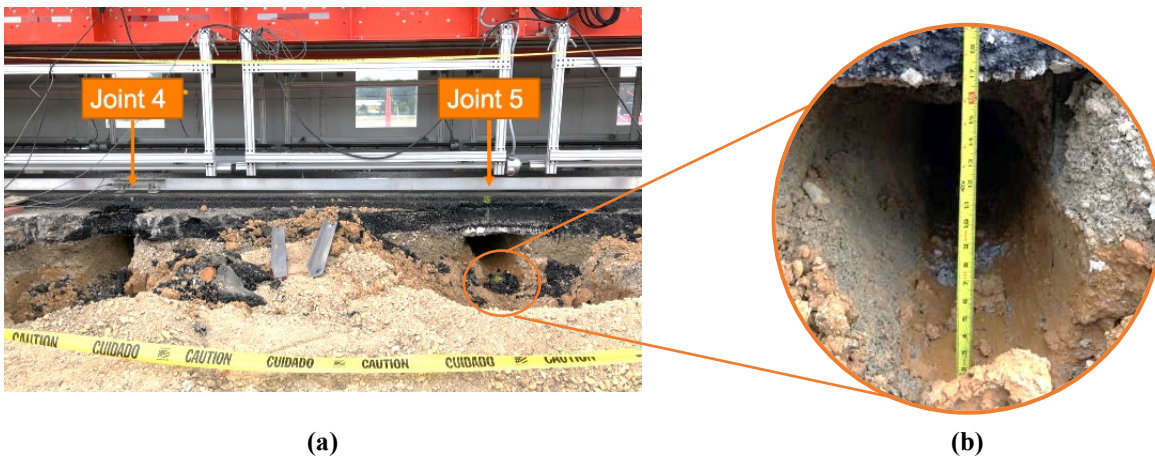
Figure 12: (a) Subbase drilling below Joints 4 and 5 with (b) an average diameter of 406.4 mm (16 inches).
