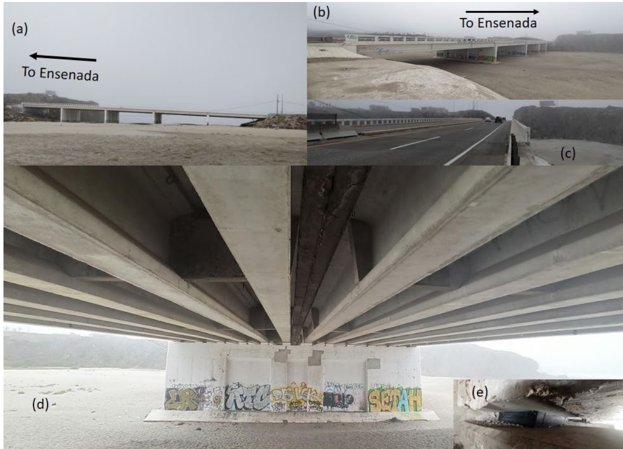
Figure 2: La Mission Bridge. (a), (b) and (c) Road view, (d) pier view and (e) neoprene plates.
